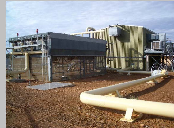
Bulla Park Compressor Coolers
