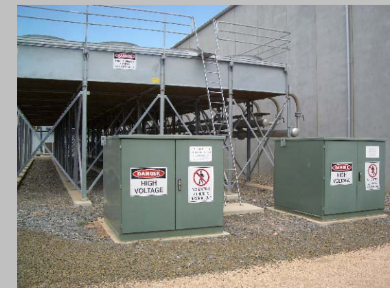
Red Cliffs Station Coolers
